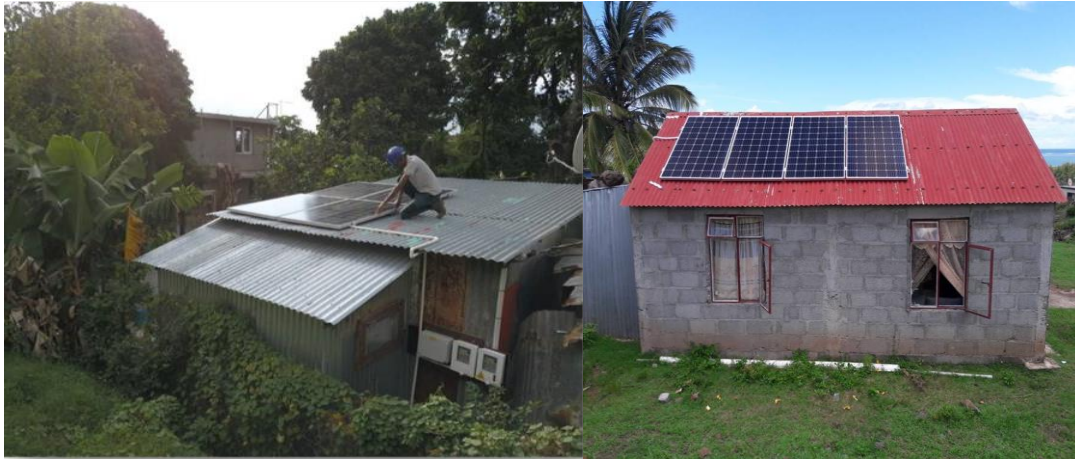
Home solar project in Mauritius and Rodrigues
