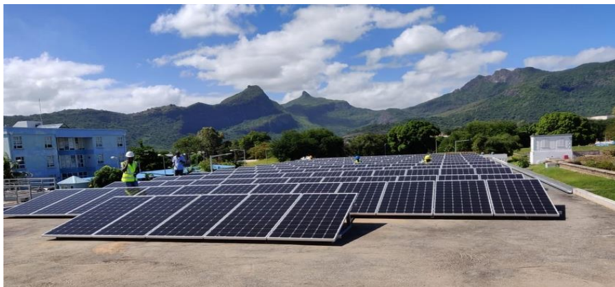
Solar system on CWA building
