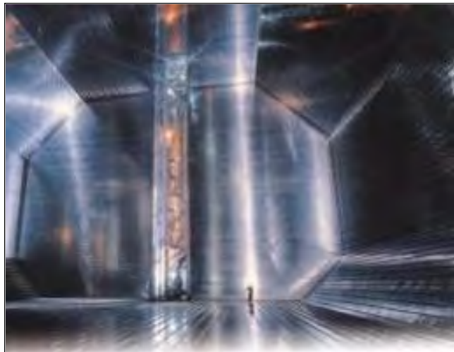
Exhibit 3-18: Membrane Tanks: Internal
