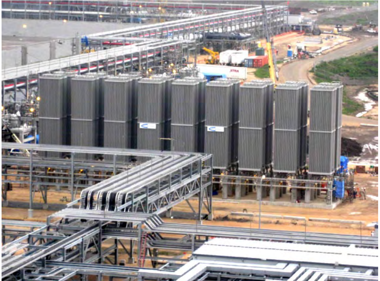
Exhibit 3-23: 200 MMcf/d (~160t/h) DAAV's at Sabine Pass LNG Terminal
